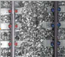
Elastic Fastener Inspection
